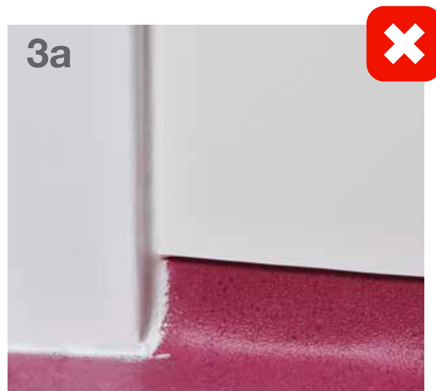
This shows a wide gap between the floor and wall sheet, and between the wall sheet and the door frame, filled with thick mastic.
