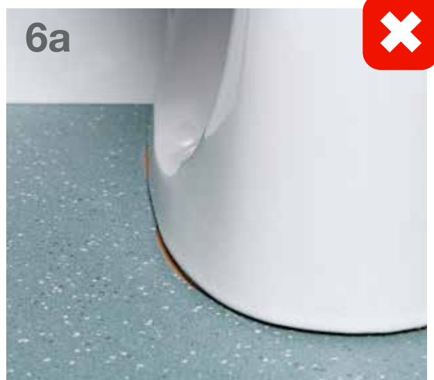
This shows a poorly cut floor with no seal between it and the toilet base.
