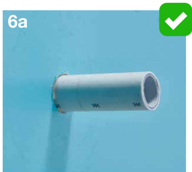
This shows a neatly cut, even sheet, with the recommended 3mm gap.
