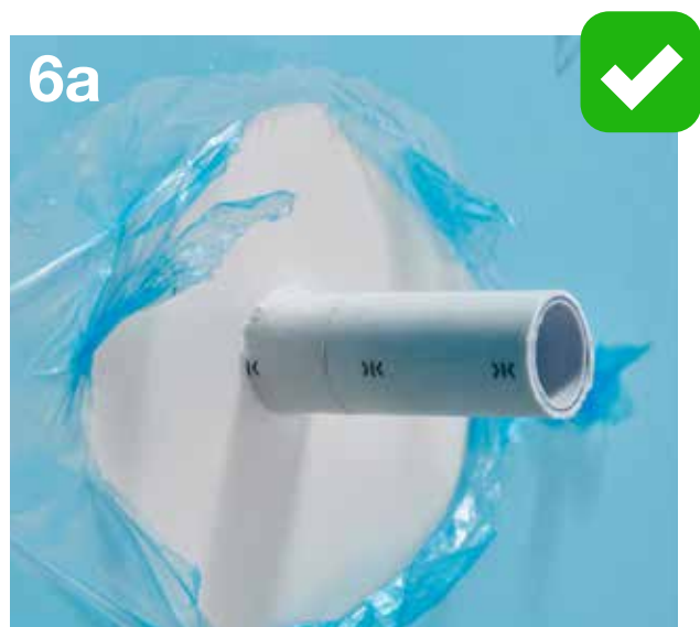
This shows pipework coming out of the wall sheet, sealed with neat mastic all the way round.
