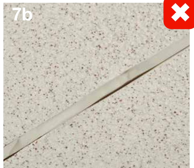
7b This shows a poor, untrimmed floor weld with gaps.
