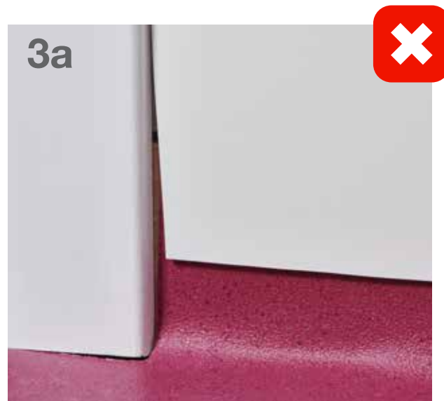
This shows a wide gap between the floor and wall sheet, and between the wall sheet and the door frame, allowing water, dirt and bugs to get behind.
