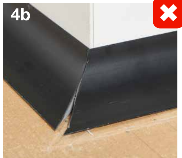
This shows a poorly cut and fitted cove former.
