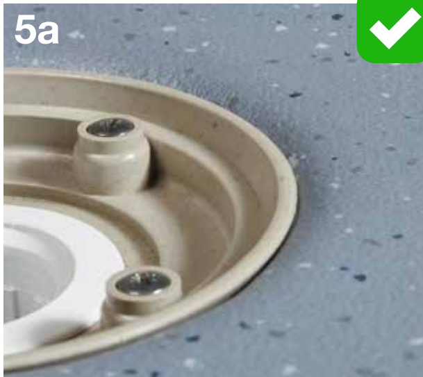
This shows the flooring folded in, with the drain fitted on top.
