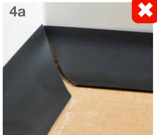
This show a badly cut and poorly fitted internal corner.
